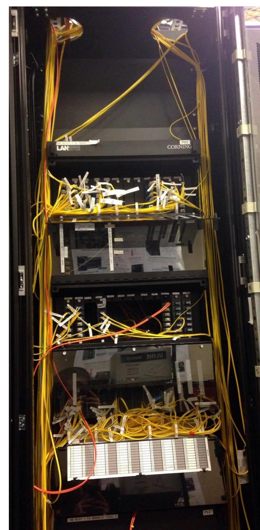
Fig 4. These optical fibers branch out from these racks to panels, and into different buildings through pipes.
