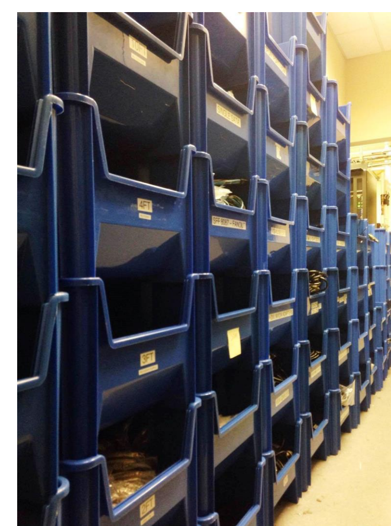
Fig 5. These bins in the PCDS server room house different components.
